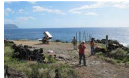
Kaena Point fence construction finally gets underway, Nov. 12, 2010. Photo by Holly Freifeld
